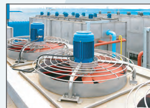
Fan and water pump
